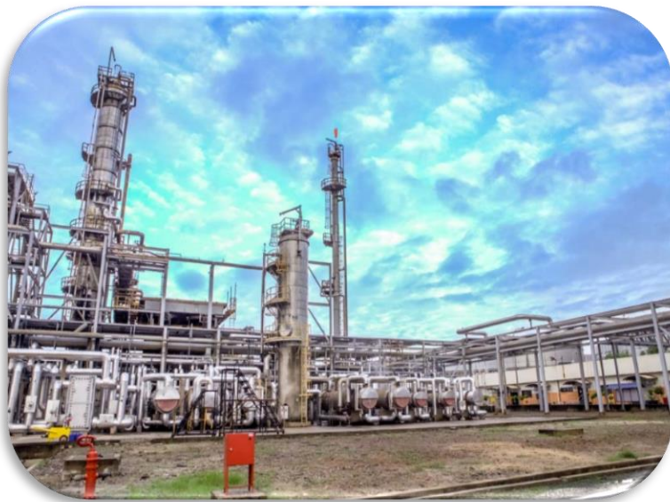
Kemaman Bitumen Plant TOMBO Rock Mineral Pipe Sections
