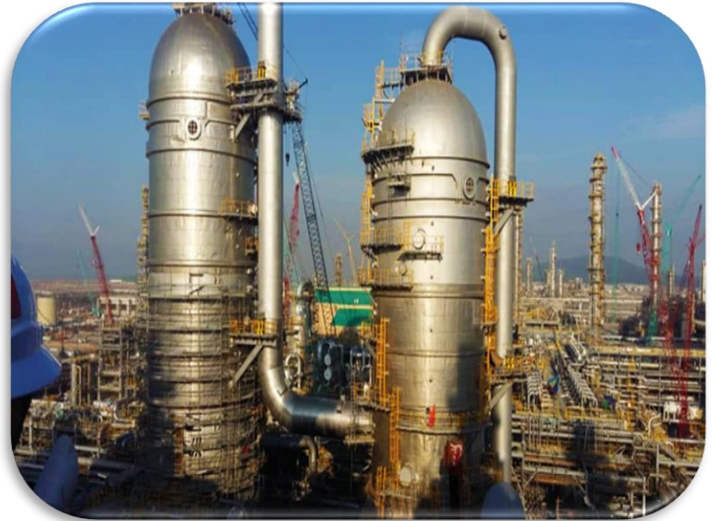
RAPID Project. TOMBO Rock Mineral Wool Pipe Cover, Wired Blanket used for Thermal Control and Personnel Protection.
